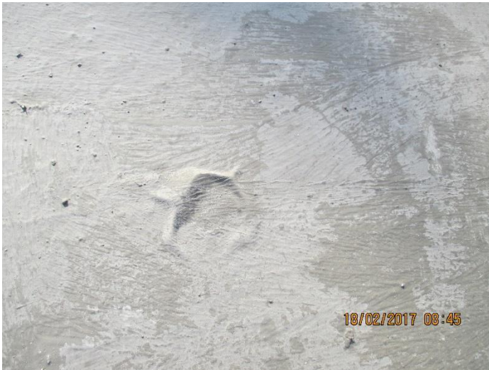
Air bubbles (Uprising moisture)
